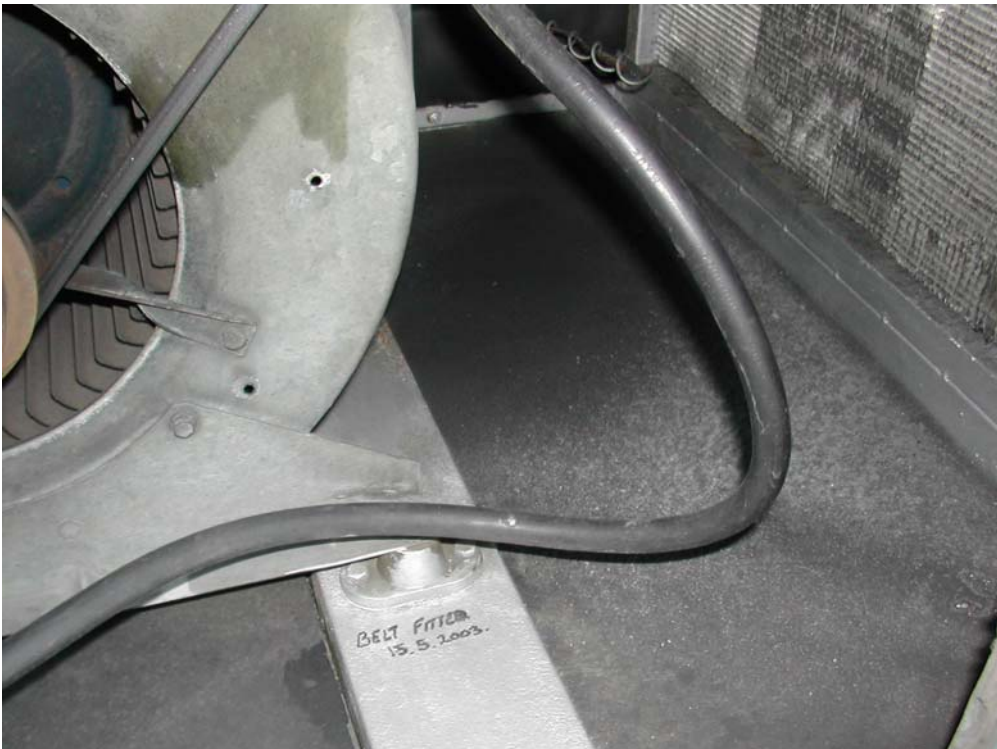
The fan chamber has heavy fouling to base.
