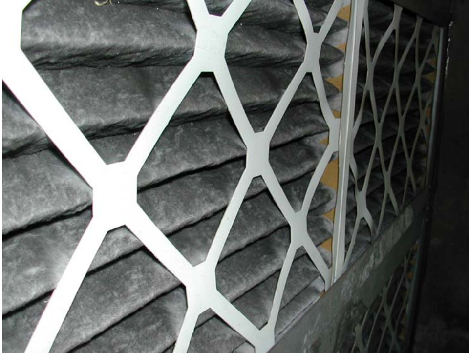
Pre- filters with light fouling.
