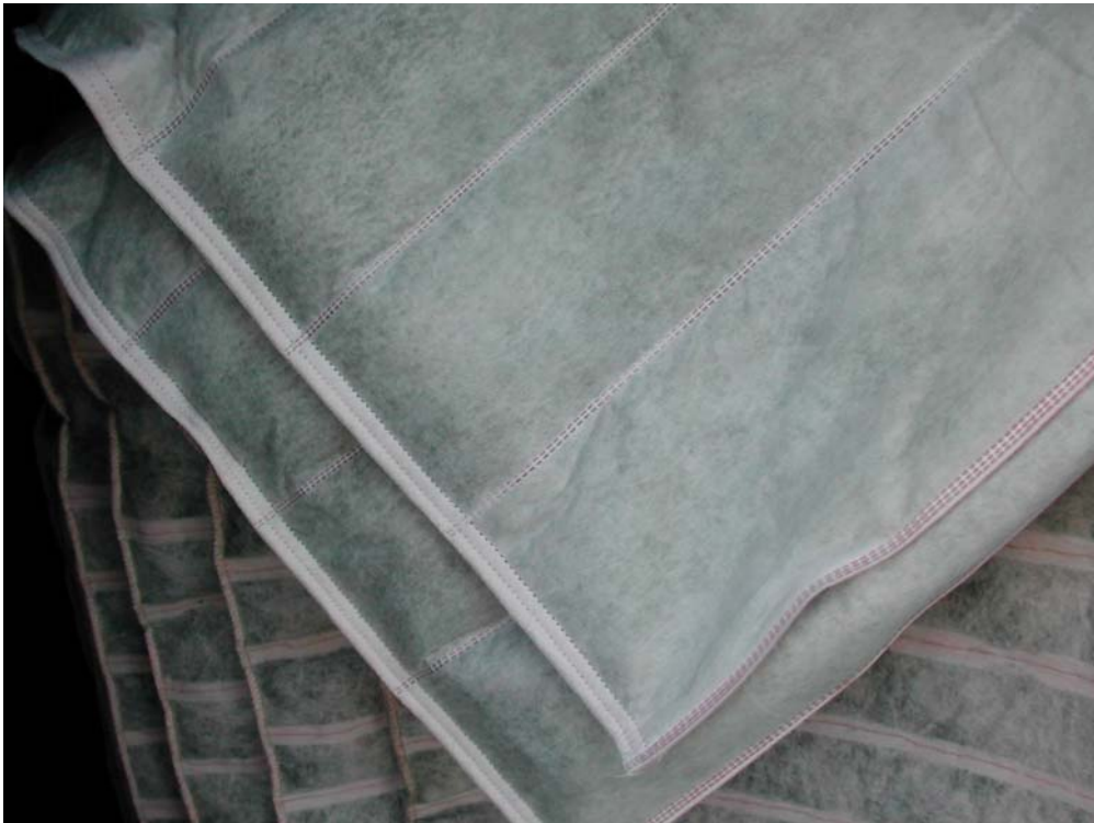
Bag filters - light fouling.
