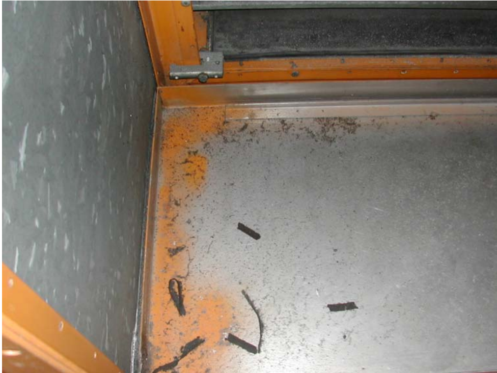
Debris within the unit including rubber fragments.
