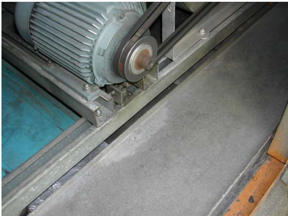
Some debris evident in the fan area.
